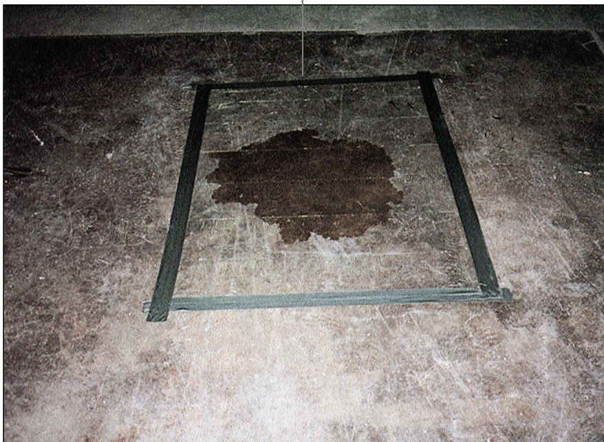
Figure 3. A plastic sheet can be used to test for moisture. Take the sheet and duct-tape it to the floor. Leave in place for 24 hours. If water is moving through the concrete slab to the surface, it's trapped by the sheet. If the coating is applied at this time, the water will form bubbles or blisters in the coating. Don't apply the coating until the slab is dry.
