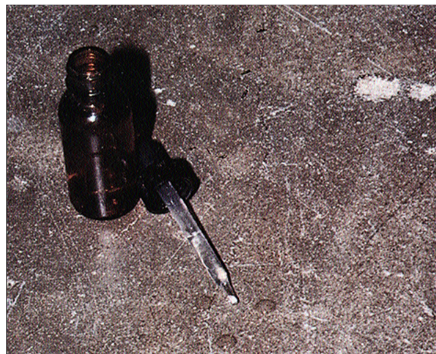
Figure 2. A water drop beads on a concrete surface if a contaminant, such as oil, grease, or curing compound, prevents the water from being absorbed. These contaminants also will prevent a coating from adhering to concrete. After surface preparation, perform a water drop quality-control test to ensure
